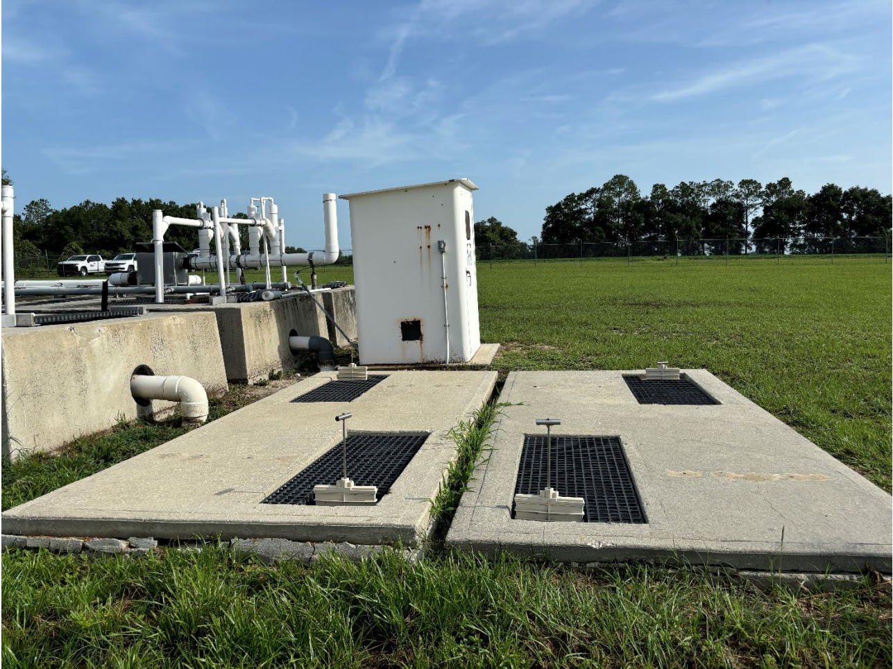
Figure 3.6 - Chlorine Contact Chambers of the Existing WWTF in Bronson
