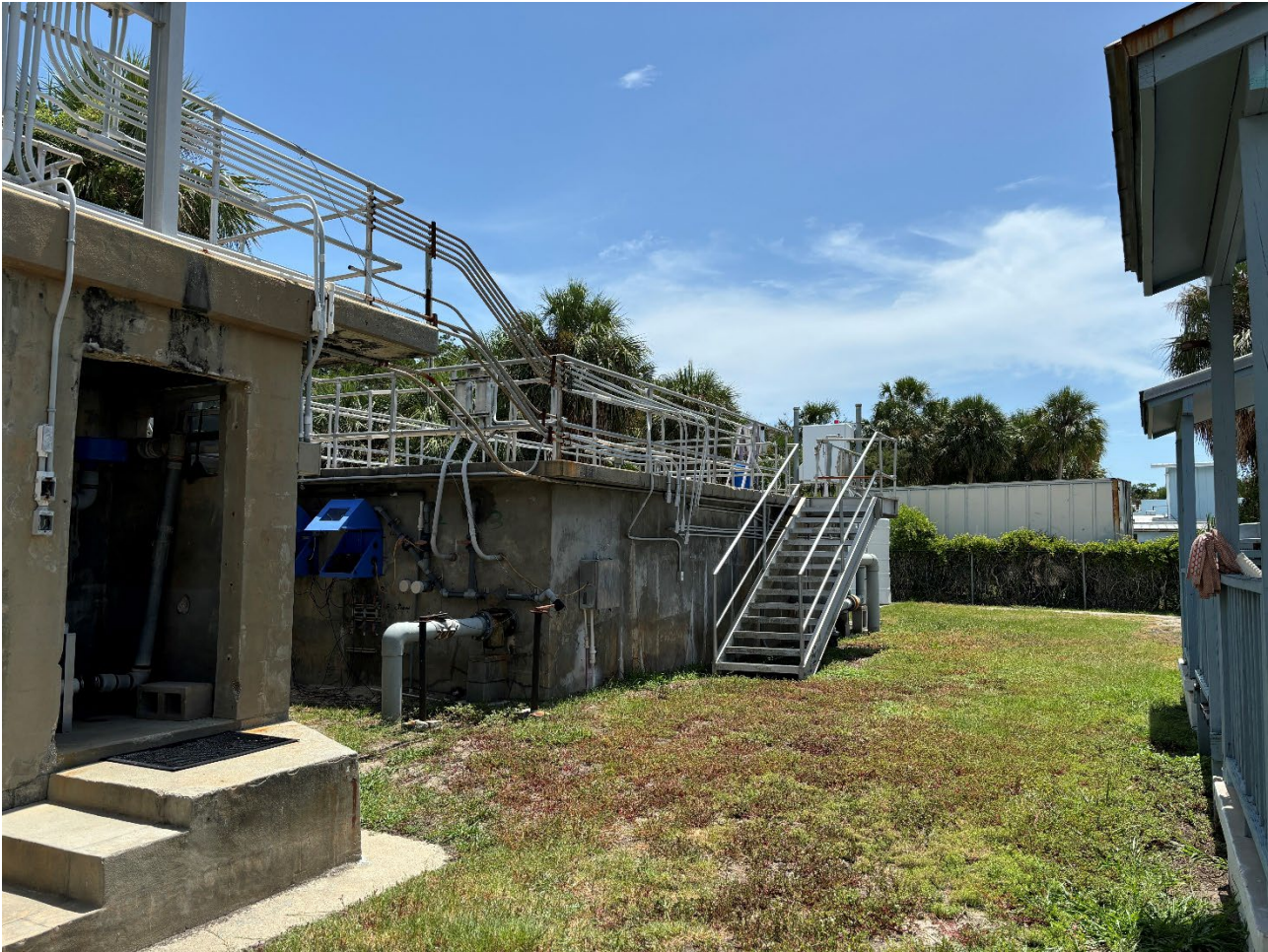
Figure 3.10 - Components of the Existing WWTF in Cedar Key
