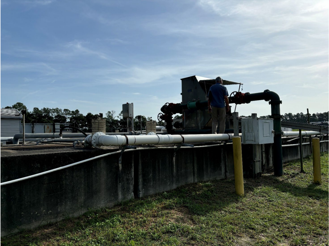
Figure 3.5 - Components of the existing WWTF in Bronson
