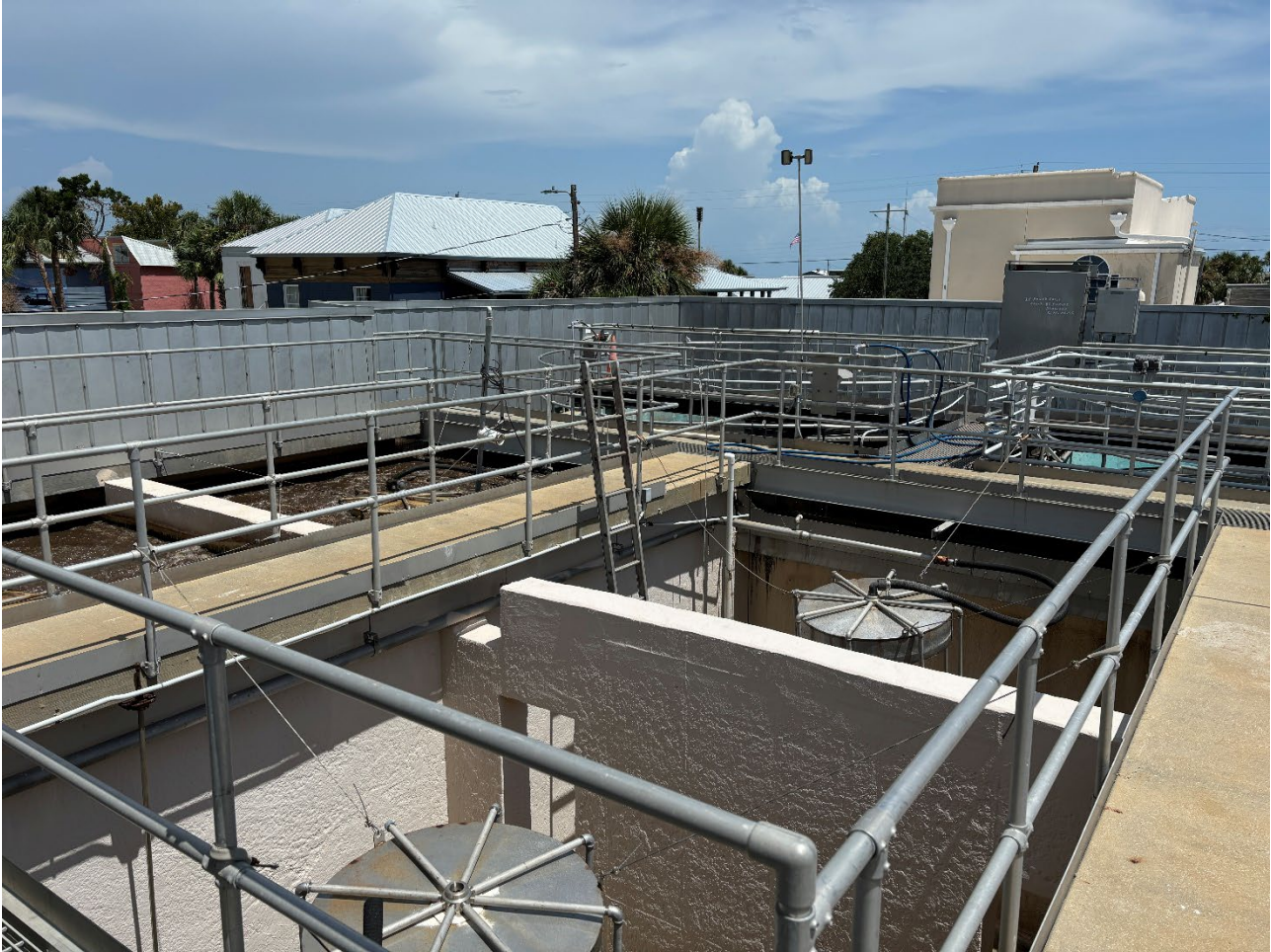
Figure 3.11 - Components of the Existing WWTF in Cedar Key
