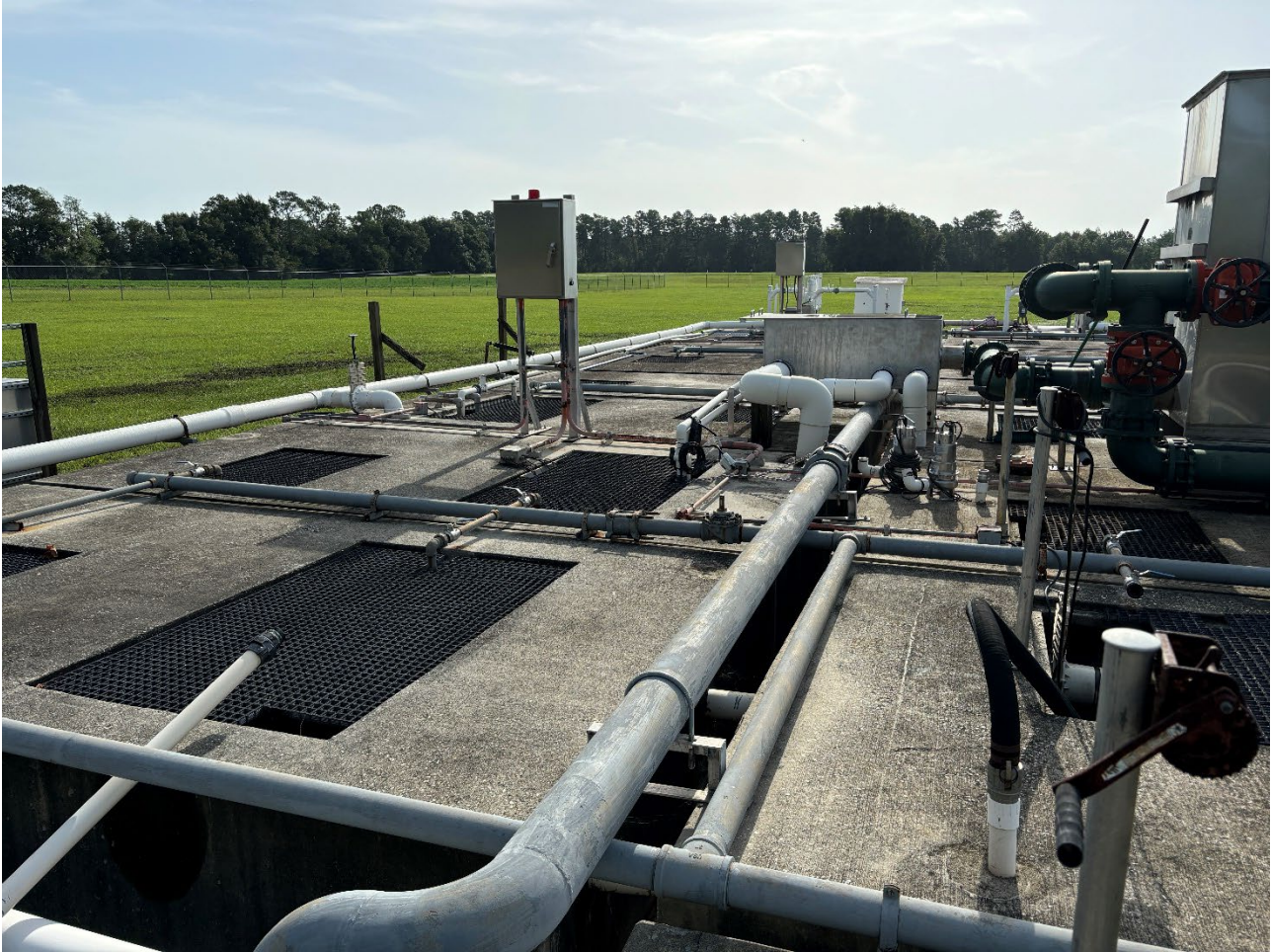
Figure 3.4 - Components of the WWTF in Bronson
