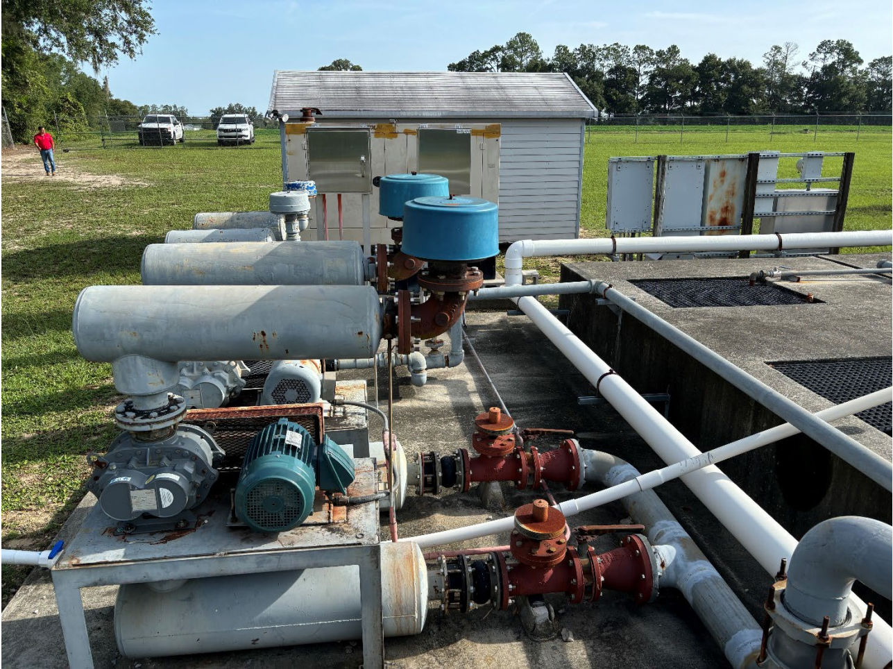
Figure 3.3 - Components of the Existing WWTF in Bronson
