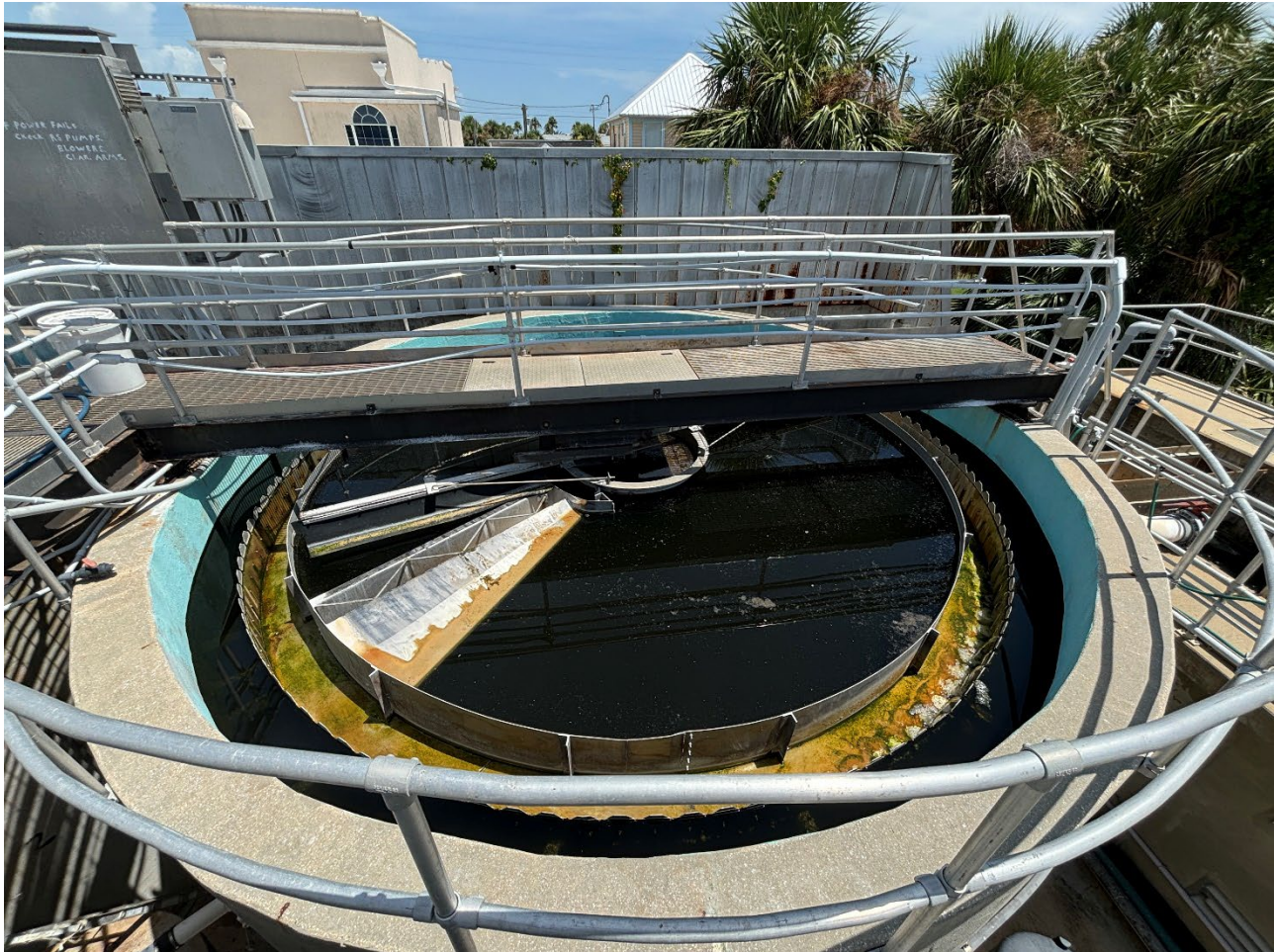
Figure 3.12 - Components of the Existing WWTF in Cedar Key
