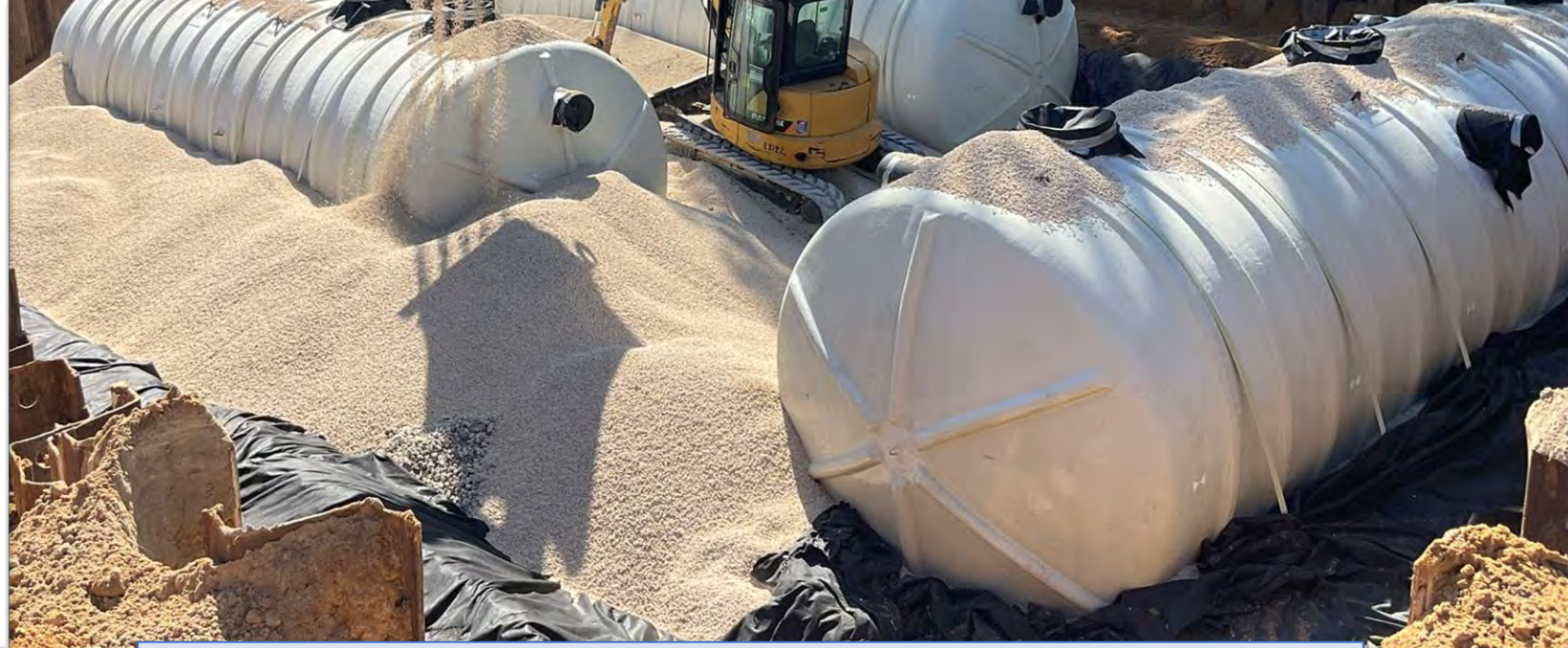
DWTU tanks (3) at 20,000 Gallons each
